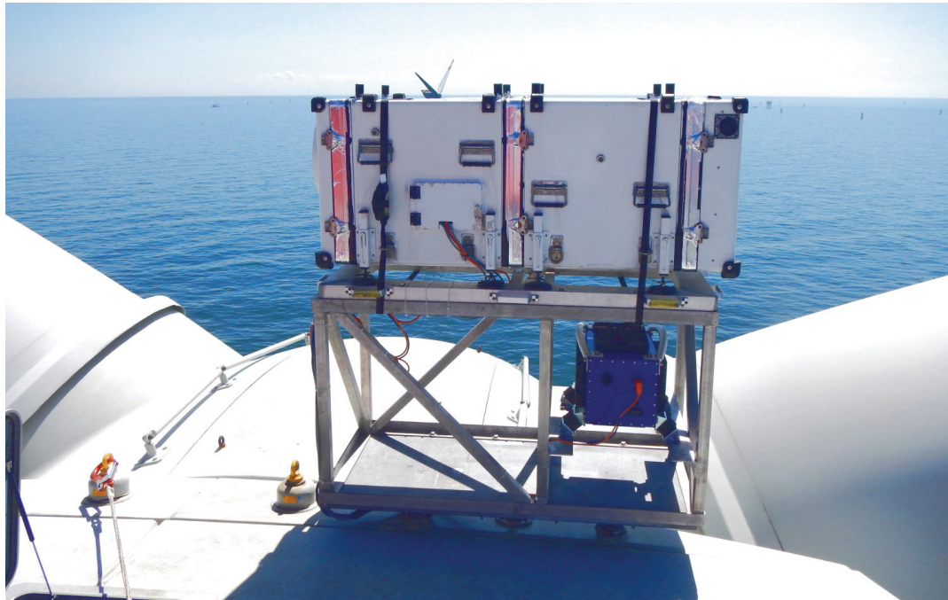
Figure 10: Lidar installation on the nacelle of a wind turbine in the RAVE offshore test field. Mounted on top of the frame is a Leosphere WINDCUBE® lidar combined with the Stuttgart Wind Energy (SWE) Scanner from DEWI GmbH, Wilhelmshaven. Whirlwind 1 is mounted in the inner frame structure on the right. Photo courtesy: Jan Anger, University of Stuttgart, Germany.
